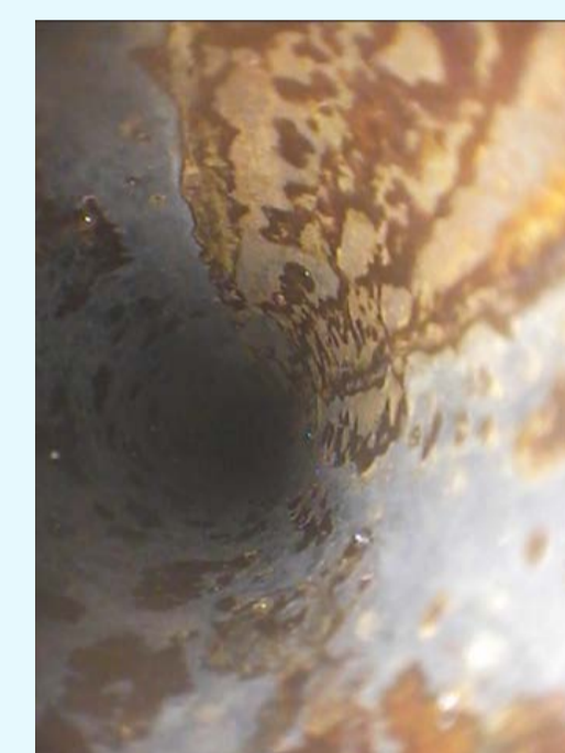
Figure 3. Surface corrosion was observed on the internal side of the tubes (all tubes were in the similar condition in time of inspection)
