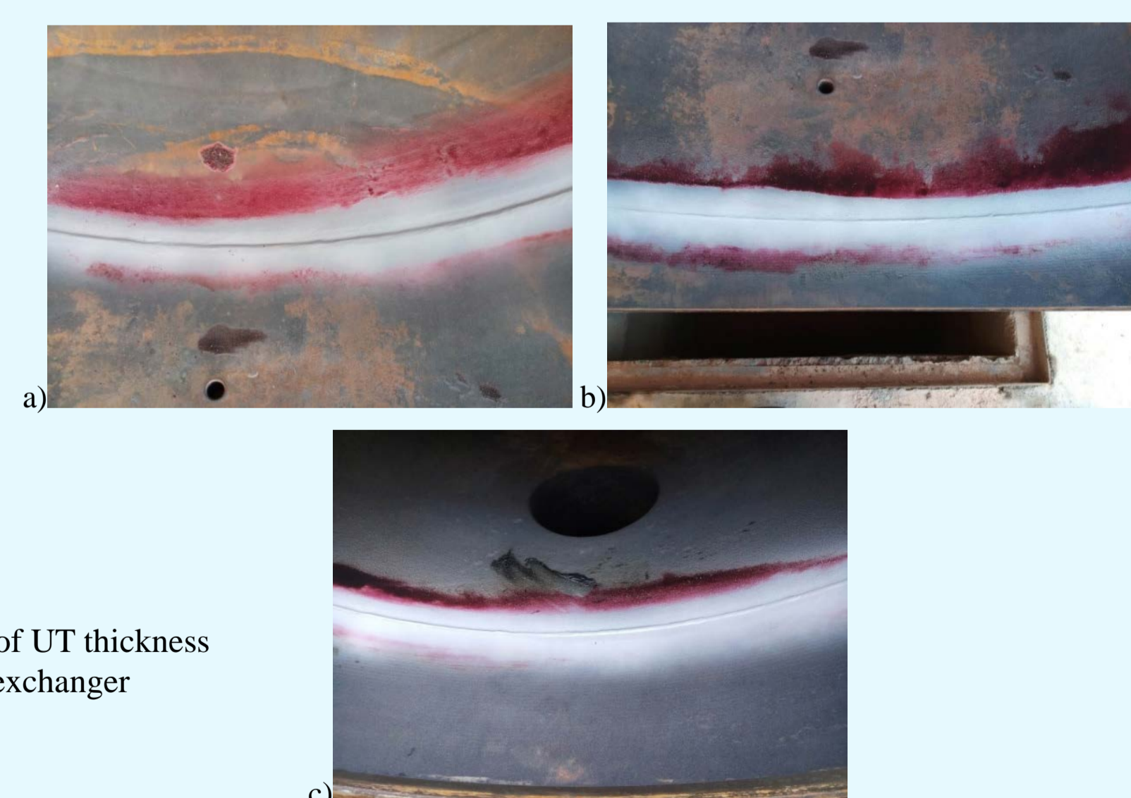
Figure 5. Results of PT tested of the weld joints a) 1 b)2 and c)6.
