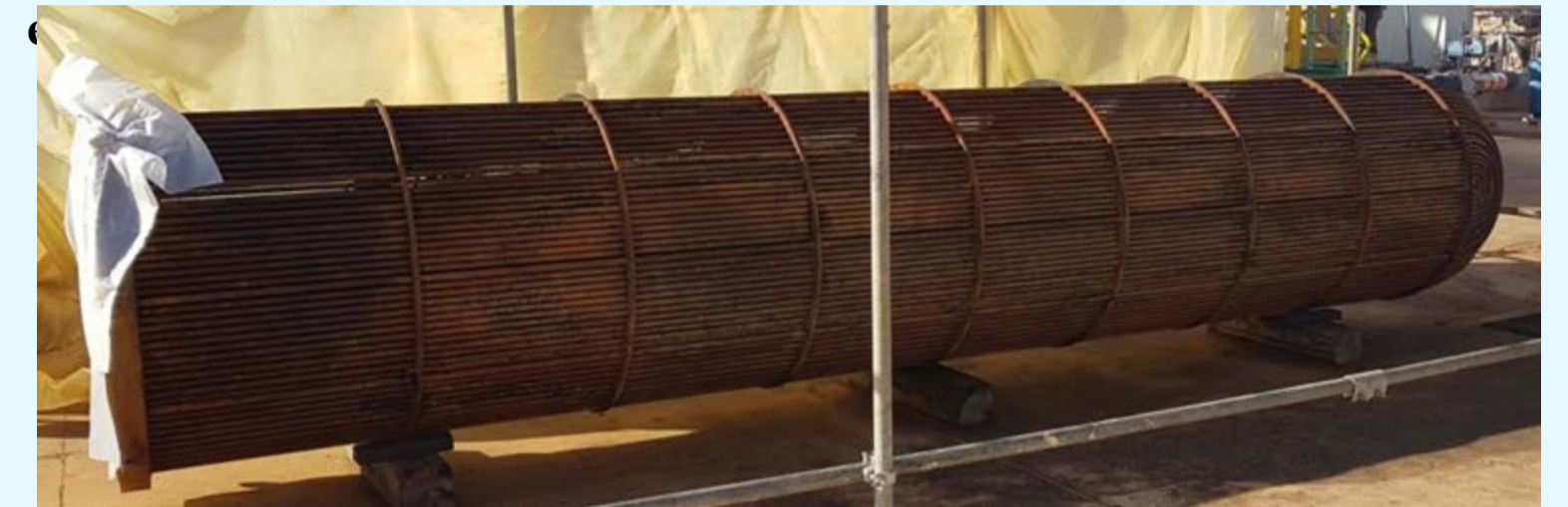
Figure 2. The tube bundle after cleaning - in good condition without visible damages and deformations
